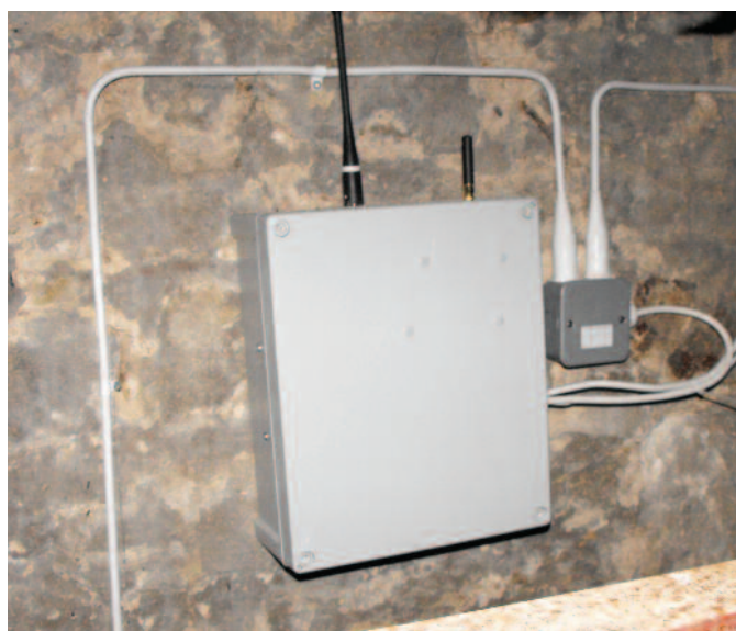
Roof security system panel installed in a church tower
